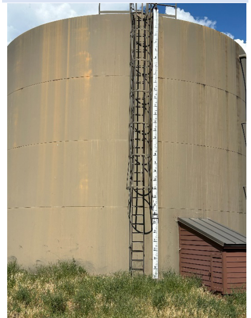
300k Storage Tank
