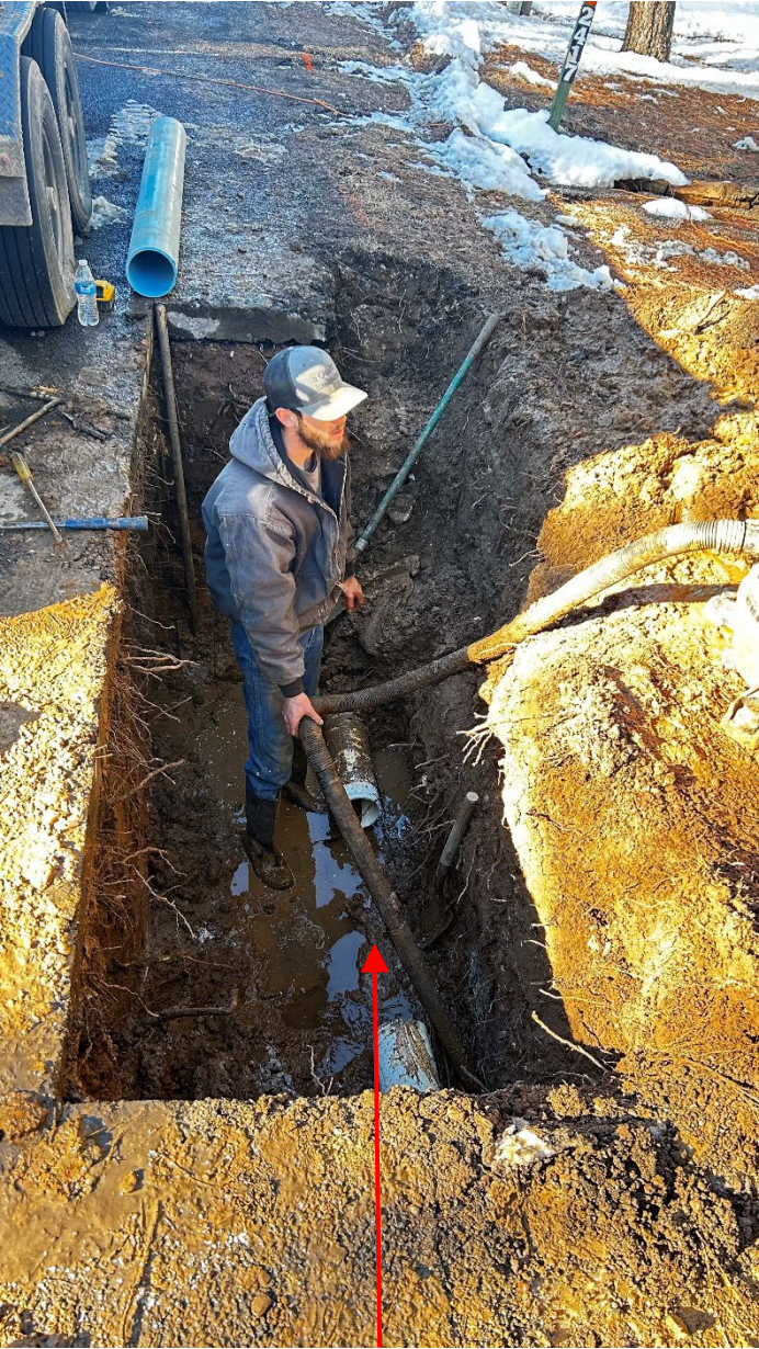
Pipe was resting directly on rock
